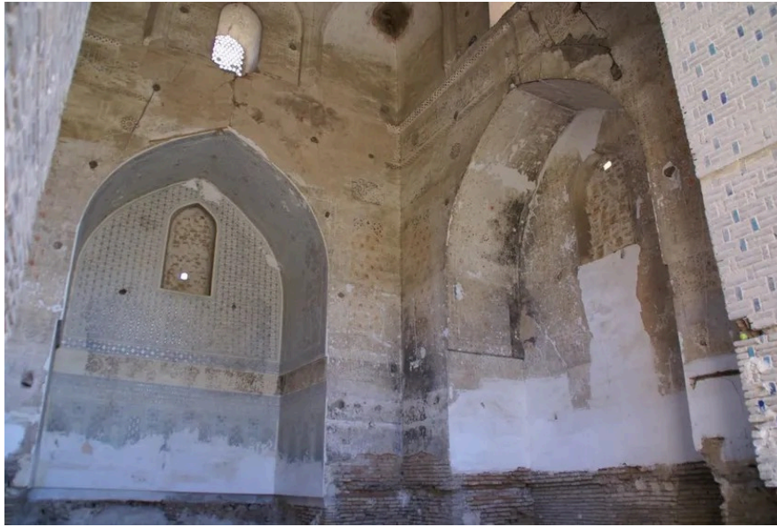
Figure 10: Interior of the southern domed chamber of the Bibi Khanum Mosque before restorations, photographed by Elena Paskaleva, 2013.
