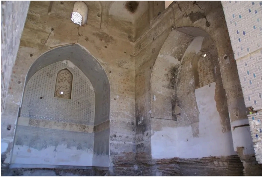
Figure 10: Interior of the southern domed chamber of the Bibi Khanum Mosque before restorations, photographed by Elena Paskaleva, 2013.
